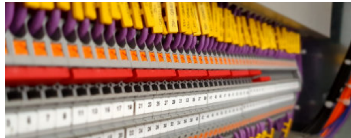
Customized secondary wiring according to customer specifications.
