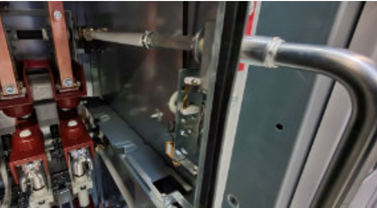
The rear right bevel gear drive ensures smooth operation of the switchgear when the door is closed. Like other manual and motor-driven actuators, it is manufactured by SZM.
