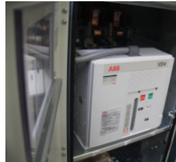
Mostly vacuum circuit-breakers type VD4, make ABB/Calor Emag (other types on request) are installed behind the front doors.
